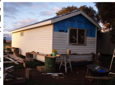
Pete has been a marvel in building our home. We only have weatherboards to put on two more walls now and then we’ll begin working on the interior: lining, decorating, electricity and plumbing.
